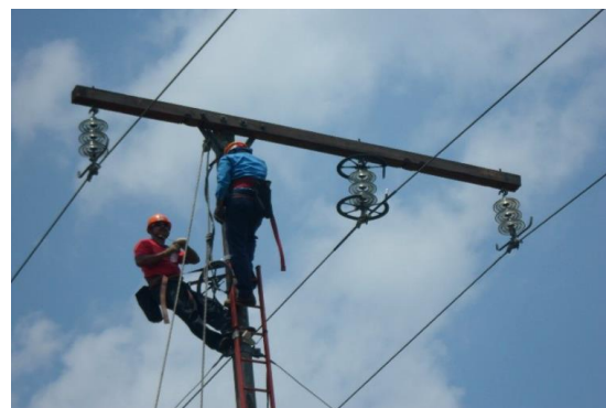
Figure 10. Installation of SAS by Malaysian DSO
