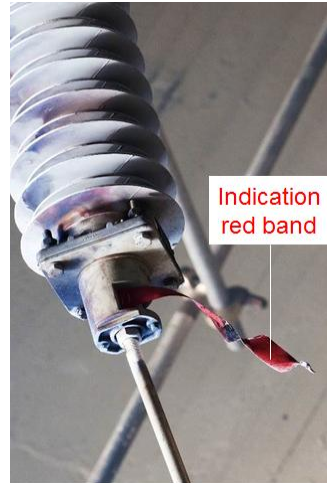
Figure 12 : Fault indicator after short circuit test. Red band must be seen properly
