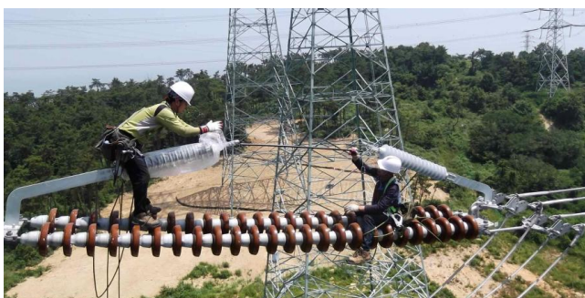
Figure 6 : EGLA KEPCO – Dead-end insulator string
