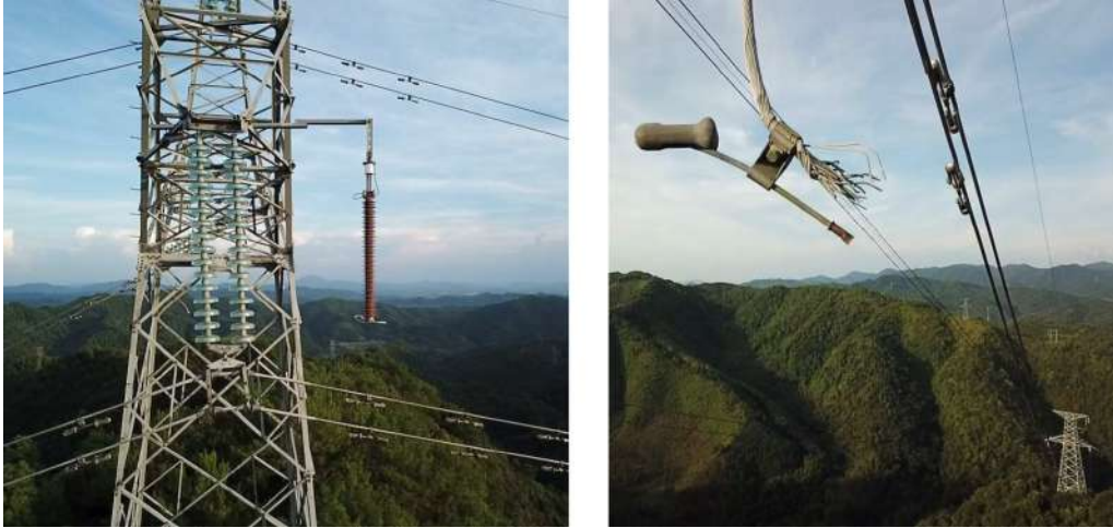
Figures 6. Damage to Overhead Conductor Due to Pressure Relief Discharge from Faulted Line Arrester (Ganzhou, China, 2017)
