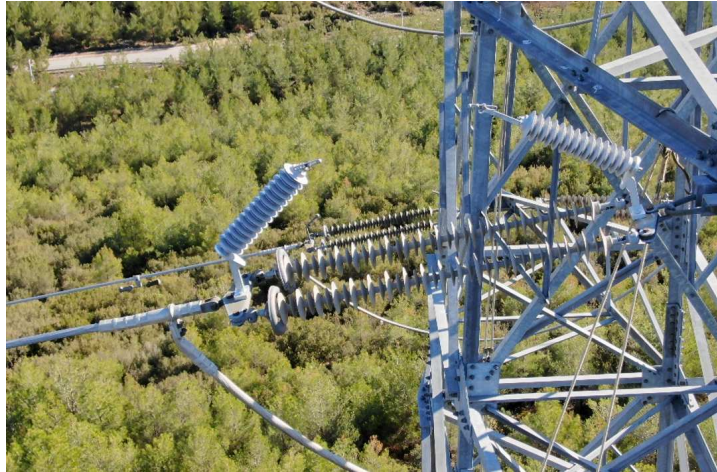
Figure 17. 170kV EGLA two body design on a double tension configuration Source: GROUND2020/21 & 9th LPE Brazil
