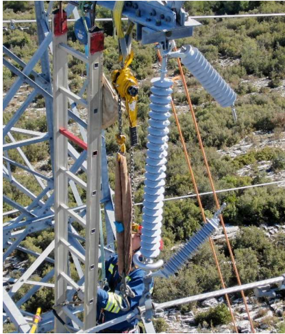
Figure 16. 170kV EGLA two body design on I-string configuration (suspension) Source: GROUND2020/21 & 9th LPE Brazil
