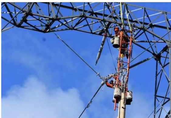
Figure 12. 230kV EGLA one body design on V-string configuration. Courtesy of NextBridge.
