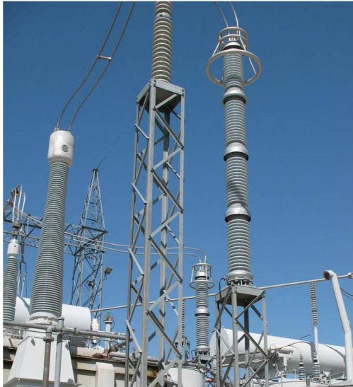
Figure 3. 500kV MOSAs at Manitoba Hydro AC-DC converter stations still in operation (installation 1979). Courtesy of Manitoba Hydro
