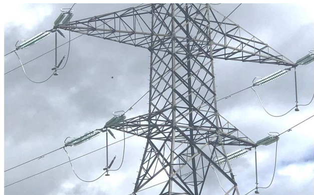
Figure 13. 230kV EGLA two body design on I-string (jumper) configuration. Courtesy of NextBridge.
