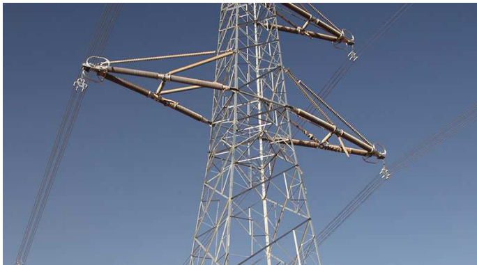
Figure 26. Example of Composite Insulated Cross-Arm (CICA) 500kV system voltage from SHEMAR
